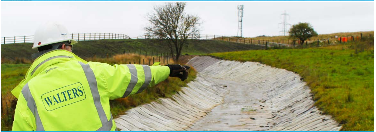
CC accommodating a turn
