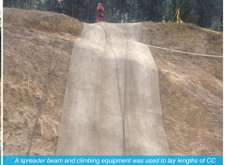
The slope prior to installation of CC, displaying signs of slip and erosion
