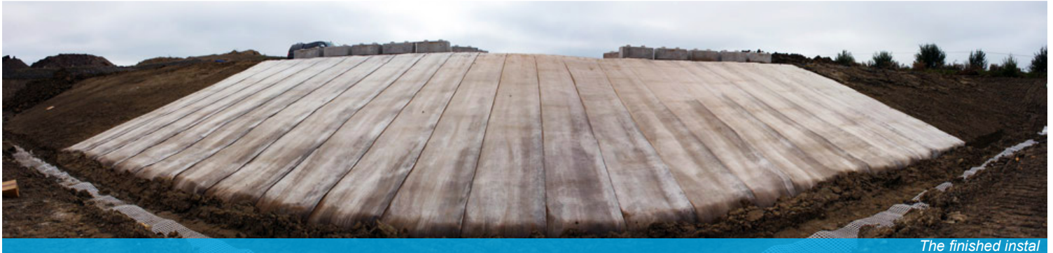
The finished instal
