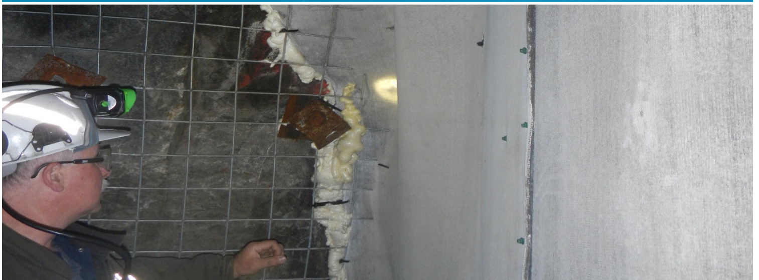
Spray foam was used to fill any voids between the vent wall and the surrounding rock
