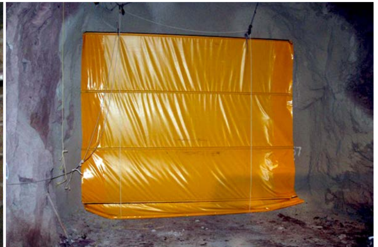
Brattice cloth had also been used but only as a temporary measure
