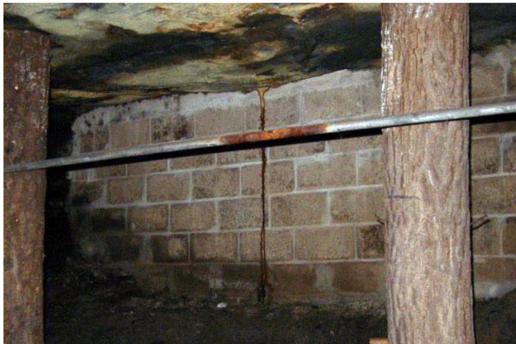
Concrete block vent walls had proved expensive and difficult to install
