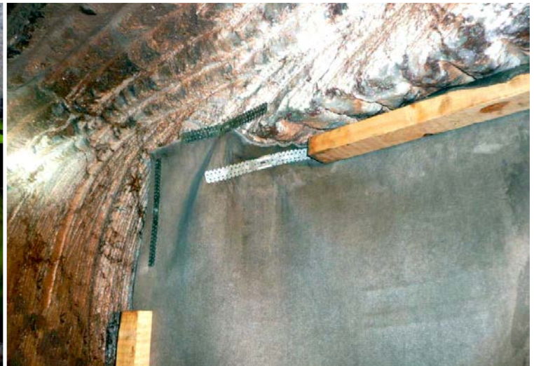
Battens, 200mm steel and screws used to provide strong fixing to rock
