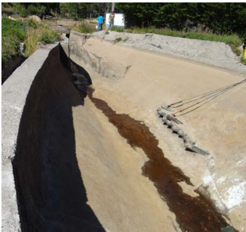
Dilapidated concrete reservoir
