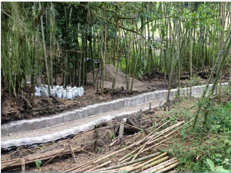
CC was applied to both sides of the 80 linear metre long ditch
