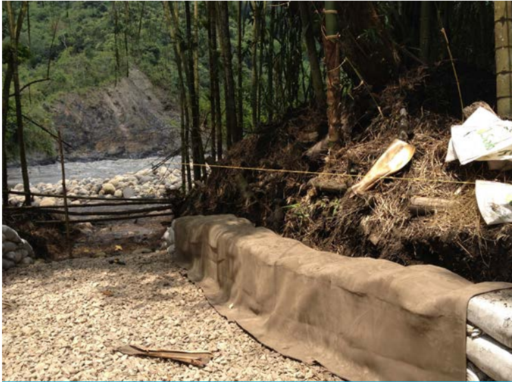
CC pre-cut sections of 1.5m positioned over sandbag wall prior to fixing
